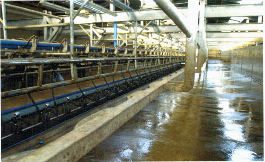
Parlour at Boreland Farm, showing Compressed Air Activated barrier (page 37). (Photo : Bob Geddes)
